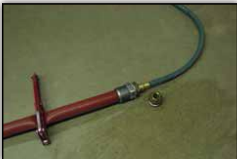
Figure 2-3. Set-up for charging the fire hose with a garden hose. The water supply is from a hose-bib (or janitor's sink) using a garden hose. The adaptor is home-made from parts available at any plumbing supply outlet. Use plumber's tape on all connections and a hose clamp to avoid leaks.
