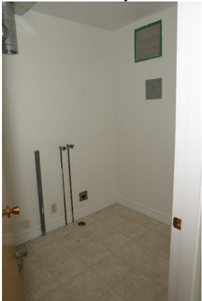
Main Floor Laundry Room
